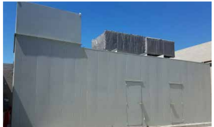
Three 2500 kW generators utilizing active CRTs with roof mounted load banks for standby power at a hospital.
