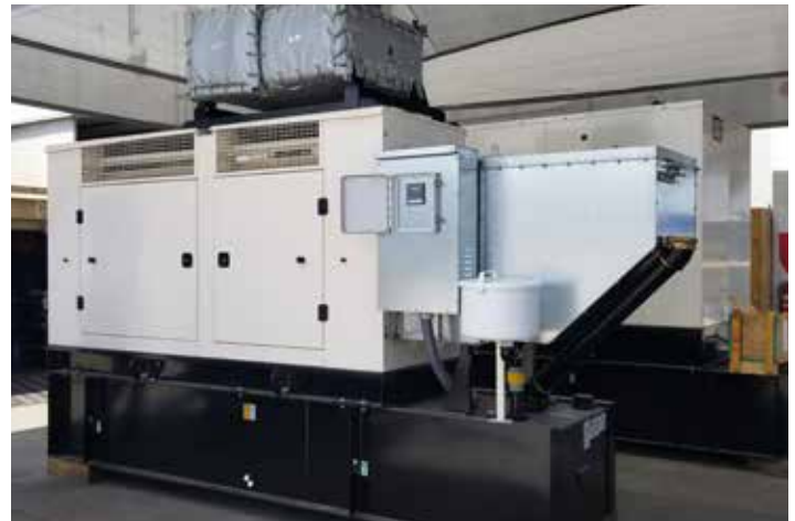
Active CRT on a 400 kW genset using 200 kW radiator-mounted load bank.
